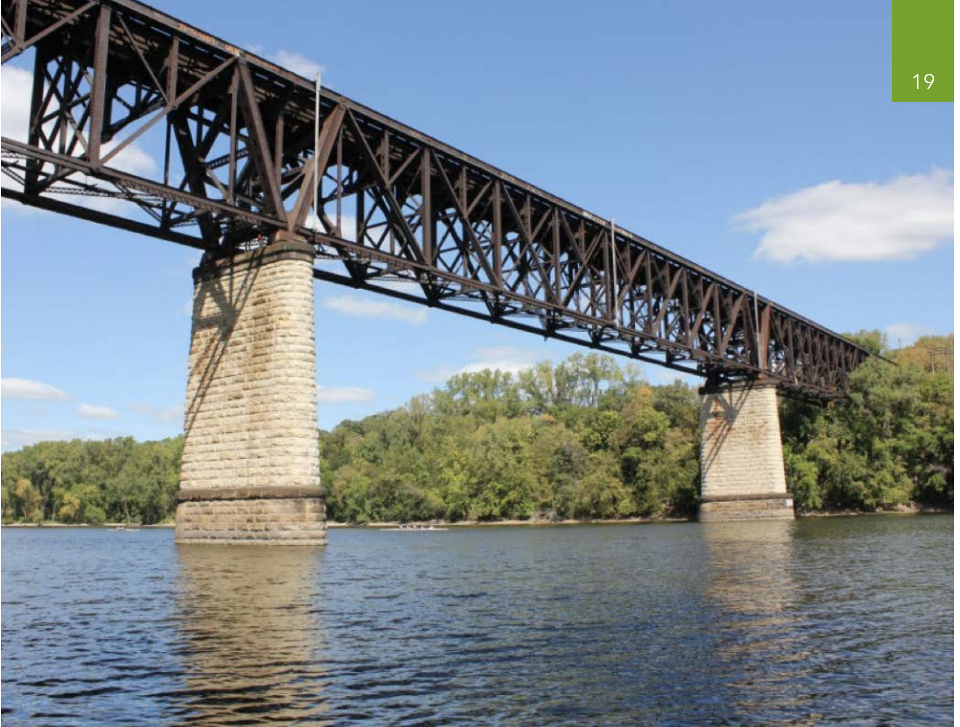
Fig. 13: Short Line Bridge - Identified as the most viable Greenway extension across the Mississippi River
