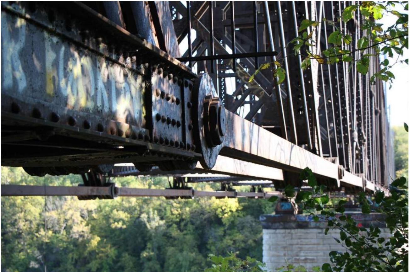
Exhibit B8: Typical lower chord pin and eyebar, south face looking east
